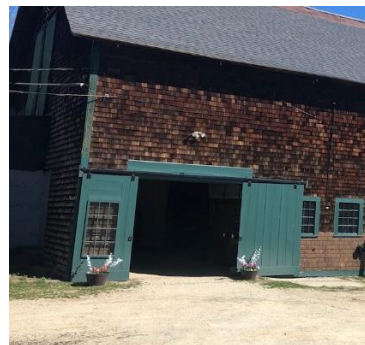
Exit 1 doors tied or secured open
